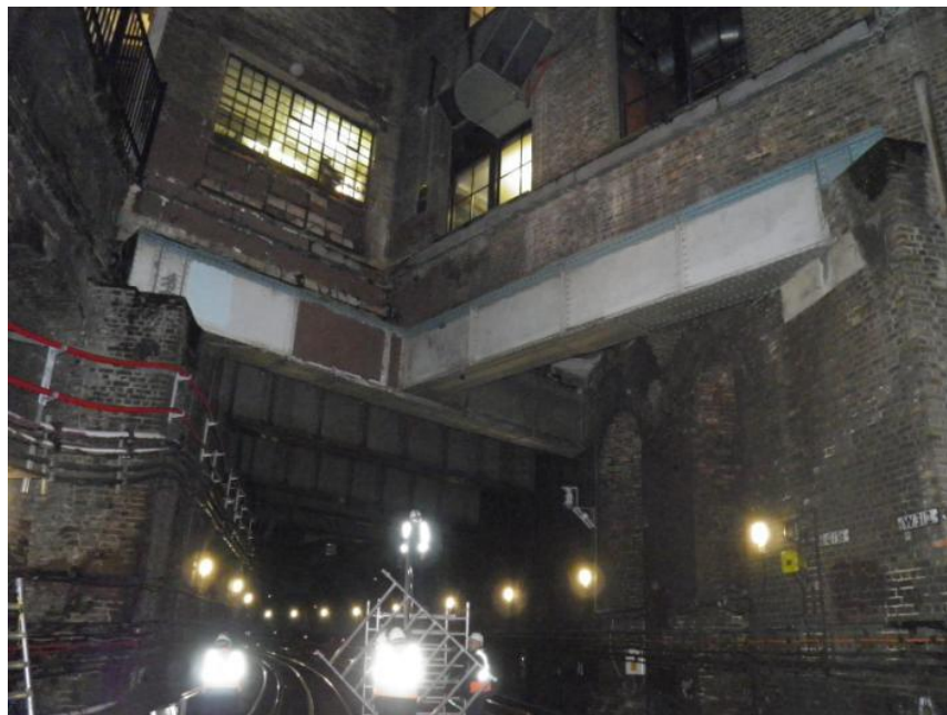
Fig.9: photograph showing girders supporting buildings, located above the Metropolitan line south of Farringdon station. Consider the primary interfaces, and how application of the conceptual framework can assist understanding of these. Source: London Underground.
