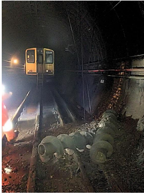
Fig.4: showing the auger on the track in the tunnel post-penetration. The service was suspended, and this train and its crew were sent to inspect the line after reports of water and debris pouring in to the tunnel by a passing passenger train. Source: RAIB, 2014.
