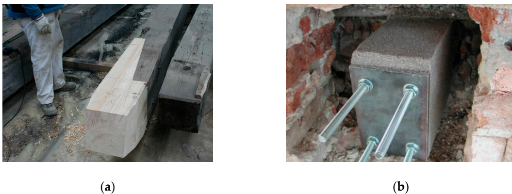
Figure 13. Re-construction of the beam ends: (a) stainless steel reinforced wooden prosthesis; (b) detail of the stainless steel reinforced epoxy prosthesis [48].
