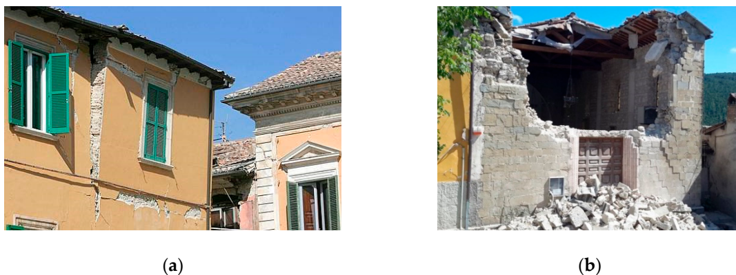
Figure 27. In seismic prone areas, wooden floors may prevent the out-of-plane mechanism of external walls (overturning). To facilitate this function, the wooden floors should be stiff enough (in-plane stiffness) and effectively connected to the walls to transfer the seismic load to the walls parallel to the seismic direction.
