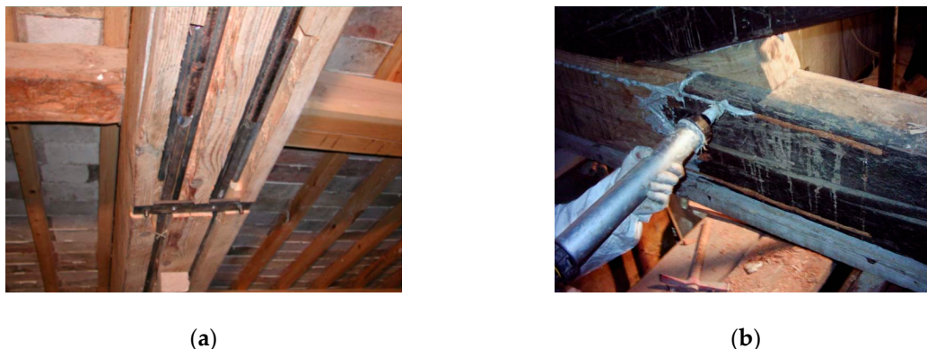
Figure 25. Bonded-in steel bar reinforcement: (a) detail of the reinforcement before resin application; (b) filling of the grooves with epoxy paste.
