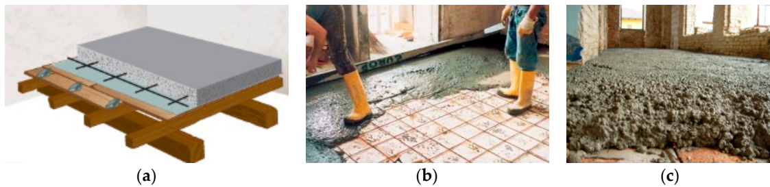
Figure 28. Traditional reinforcement of one-way wooden floor. A steel mesh reinforced concrete slab is applied over the wooden floors (there are no connections between the slab and the timber beams or rafters): (a) schematic arrangement; (b) RC slab application; (c) use of autoclaved aerated concrete; to reduce the RC slab weight (dead loads).
