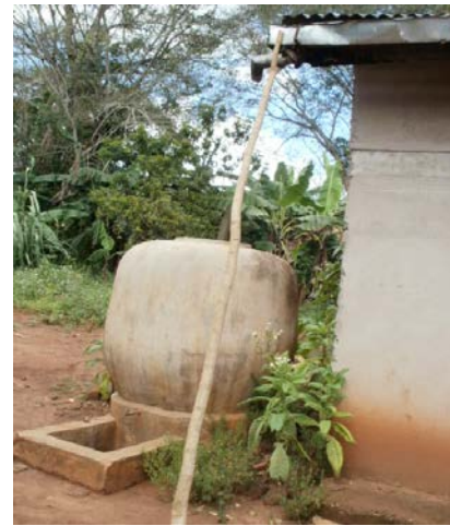
Figure 4. Tank for rain water harvesting
